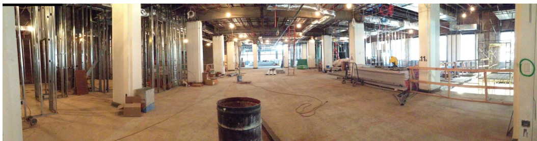
Third Floor Job Center, Computer Lab and Library Staff Work Areas on 3rd Floor
